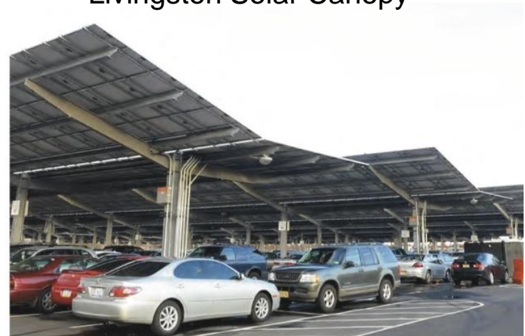
Livingston Solar Canopy
